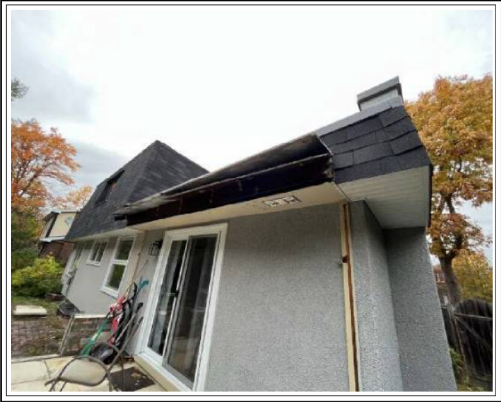
damaged soffit/fascia where solarium was attached
