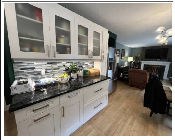
kitchen / hardwood separation seam
