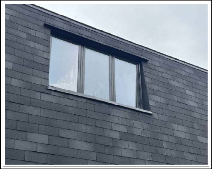
some windows have signs of condensation
