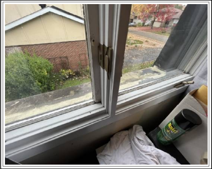
original windows / reported leaks in some storms
