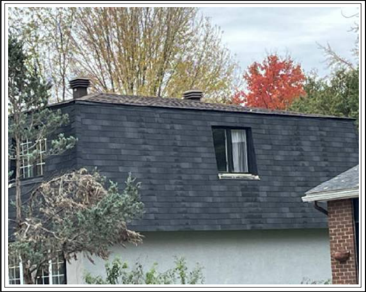
side roof shingles replaced top portion / different colour /roof shingles appear to curl
