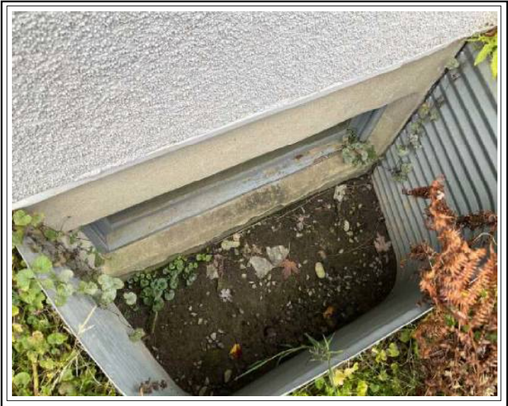
windows well requires maintenance wood basement window / signs of water damage
