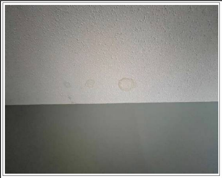
dining room ceiling / signs of water damage
