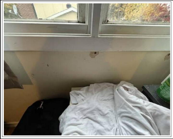
drywall under window damaged / signs of water damage
