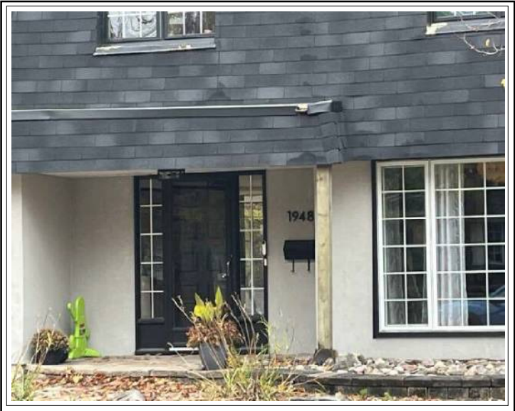
roof over hang unlevel
