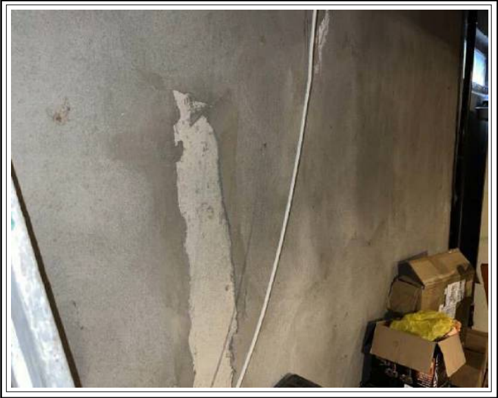
interior basement parging missing
